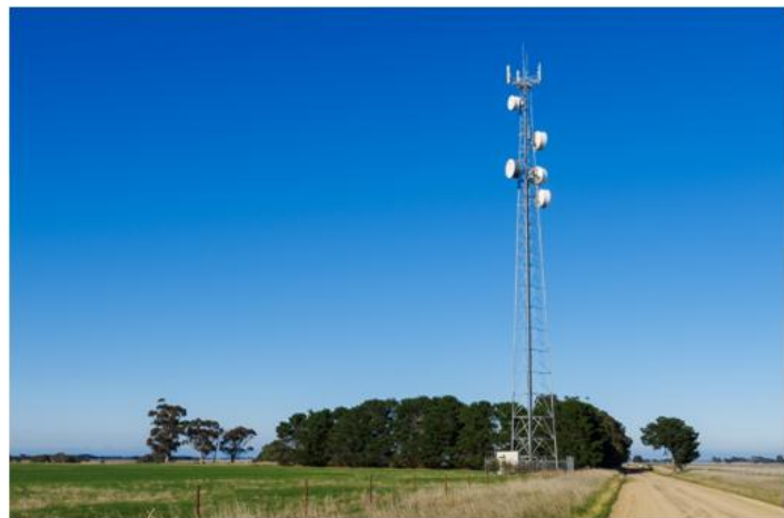
Figure 2 High-Mounted Fixed Service Antennas Source: Carl Chapman Photography. With permission
